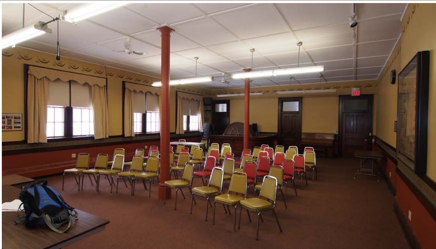
Central core – Banquet hall showing steel columns. Wood beam carrying second floor structure is above lowered ceiling.
